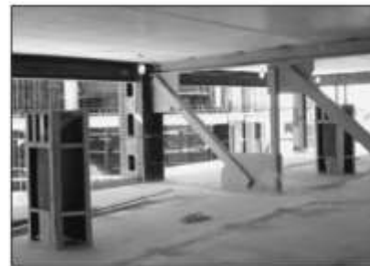
Staggered steel trusses, floor to floor in depth, support hollow core slabs in new Marriott Hotel in Hartford, CT. Slabs provide instant work platform for other trades as shown above. Photo by Corley
